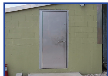
Mechanical Room Flood Door (PD-525)
