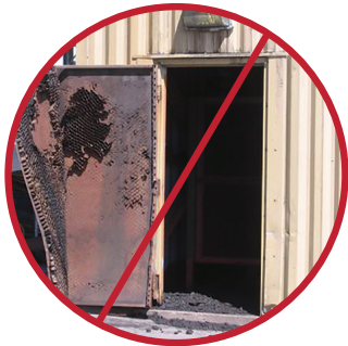
Failed Hollow Metal Door
